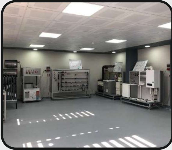
AMASYA ŞEHİT GULTEKİN TIRPAN VOCATIONAL AND TECHNICAL ANATOLIAN HIGH SCHOOL INSTALLATION TECHNOLOGY AND AIR CONDITIONING WORKSHOP
